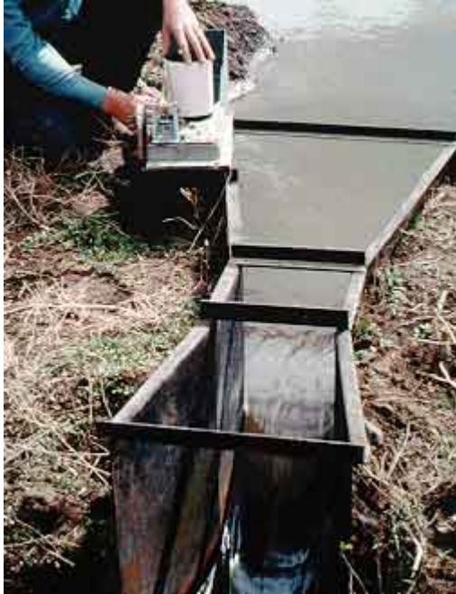
Figure 5: Parshall Flume Installed in a Channel
