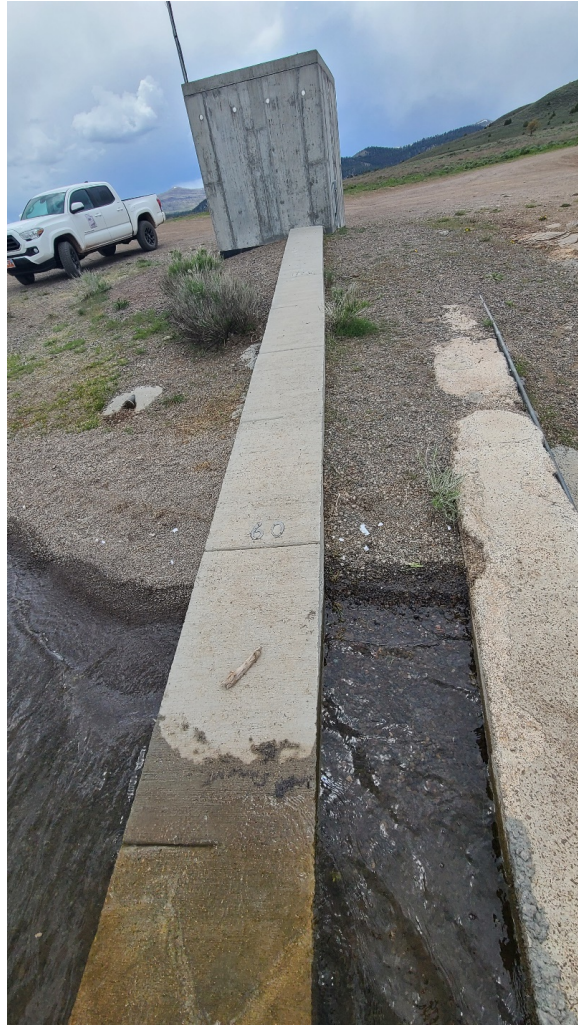
Caption: Staff gauge and outlet control building.
